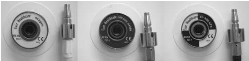
Figure 1.1 – Wall-mounted outlets and gas-specific probes for (left to right) oxygen, nitrous oxide, air
