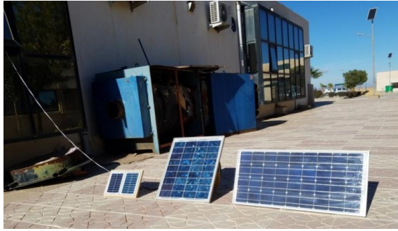
Fig. 8 – PV modules installed, three panels were used
