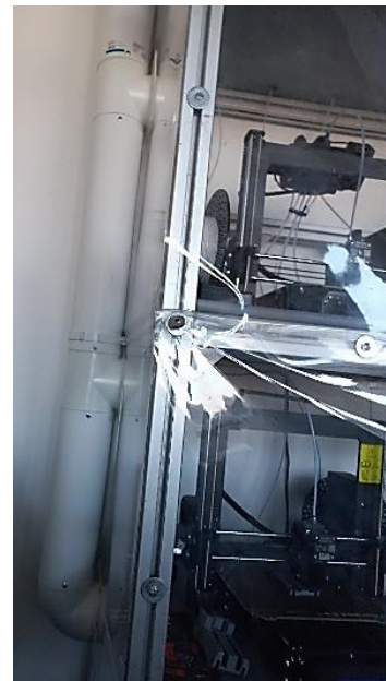
Figure 3 – A ventilation shaft for the removal of dangerous gases and maintaining a stable temperature mode
